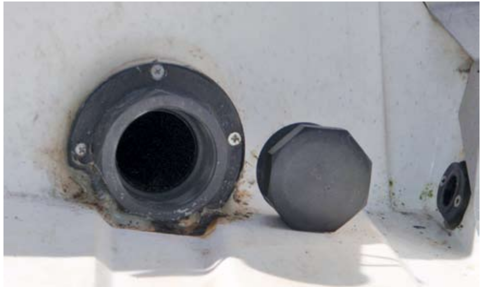
Inside the hull, 60mm Hansen's fittings have been used so Geoff can close off the scuppers.
